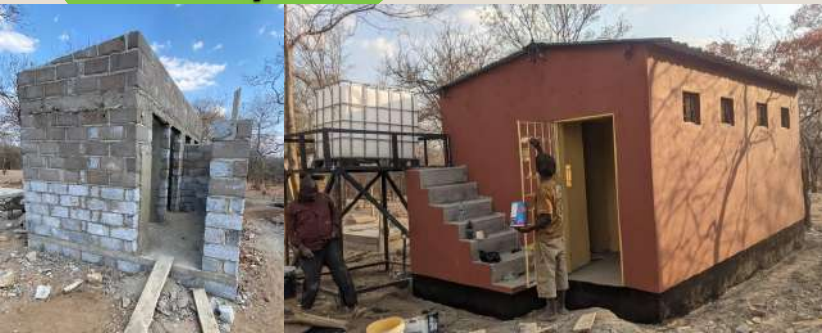
Construction of water borne ablution block at malilangwe primary school for Nyimba Town Council.
