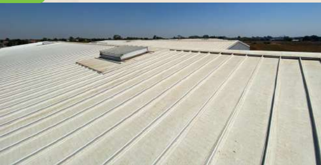
Removal and new installation of cold room roofing sheets at York park commercial park.
