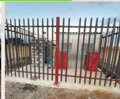
Borehole concrete slab and fencing at Coca-Cola Lusaka west plant
