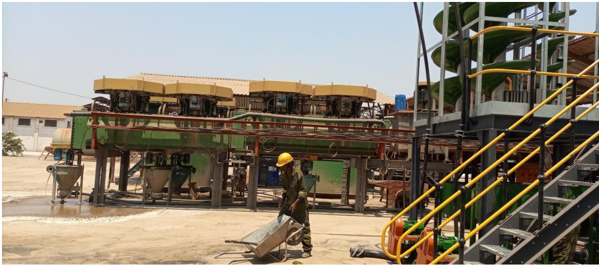
Figure 1 Showing installations of mine processing plant at Sable Zinc – civil and mechanical works done by PCA Civils
