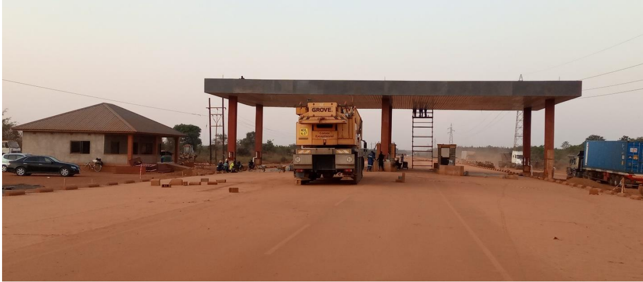
Figure 7 Toll Gate infrastructure carried out by PCA Civils for the Road Development Agency - RDA
