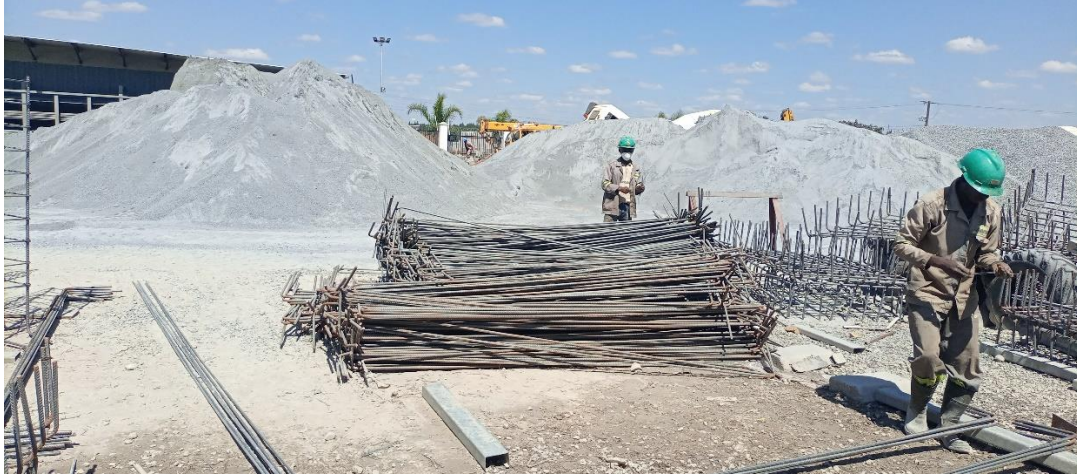
Figure 3 Preparation for Civil Works at the 120TPH Copper Concentrator at Bwana Mkubwa Ndola for Jubilee Metals Zambia
