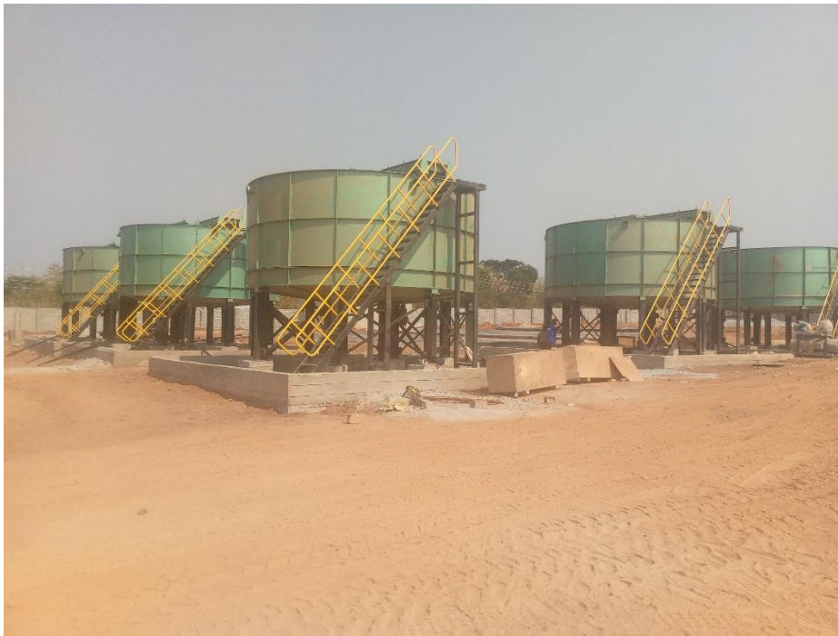
Figure 4 Civil and Mechanical works at Buntingwa Copper/Cobalt Processing Plant at Ganeton Kitwe for Buntingwa Resources
