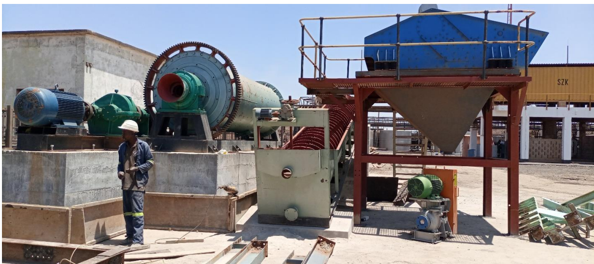
Figure 2 Showing installations of mine processing plant at Sable Zinc – civil and mechanical works done by PCA Civils
