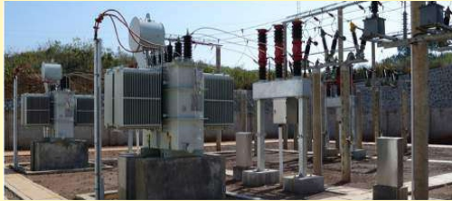
Complete Sub Station
