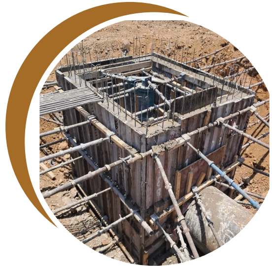
Air Valve Chamber
