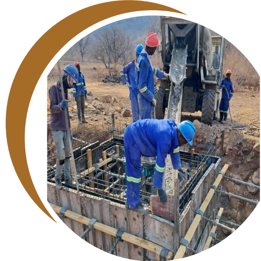
Scour Valve Chamber
