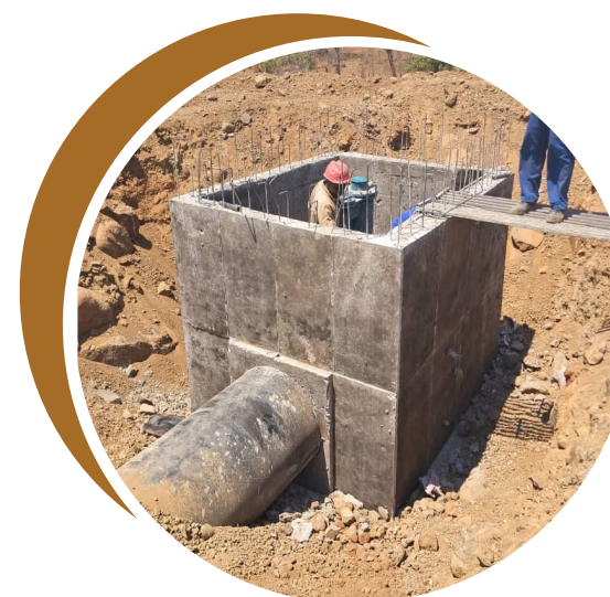
Scour Valve Chamber
