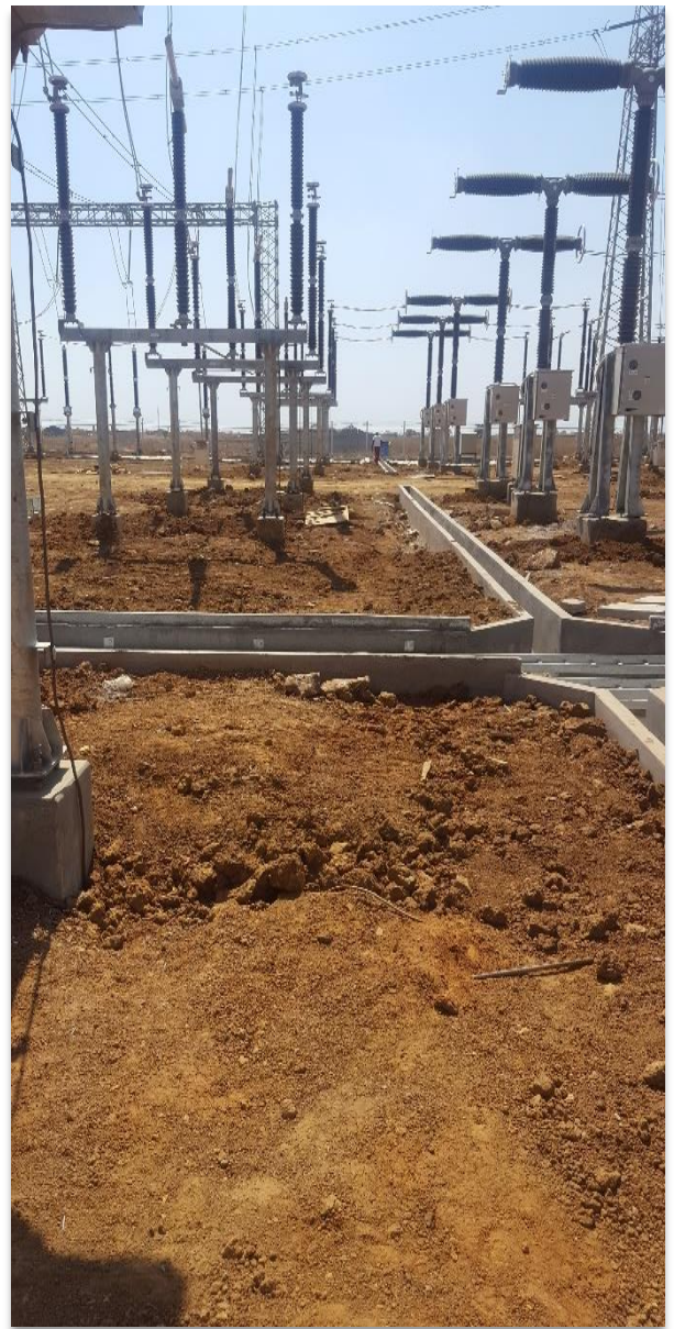
CABLE TRENCHES ZESCO LUSAKA WEST SUBSTATION
