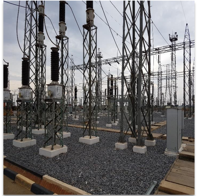
SUPPLY ON 20MM to 40MM STONE AT LUSAKA WEST ZESCO SUBSTATION 8000 TONS
