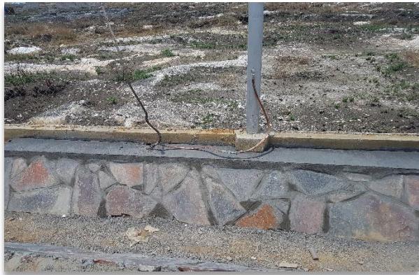
DRAINAGE AT ZESCO SUB STATIONS
