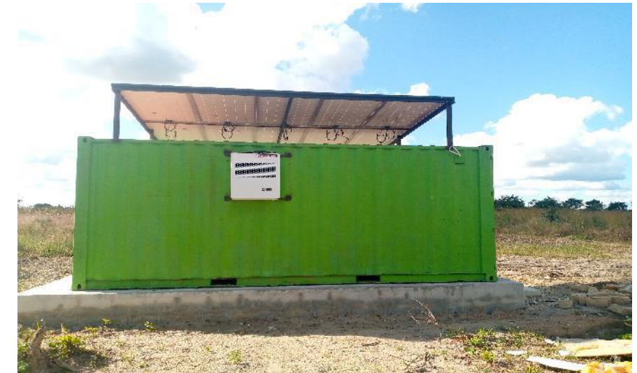
Solar Cold-Room at Kanakantapa - Chongwe
