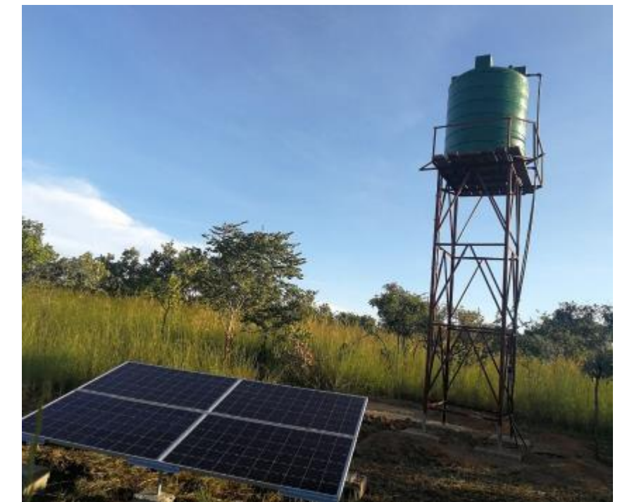
Picture of Solar Water tank
