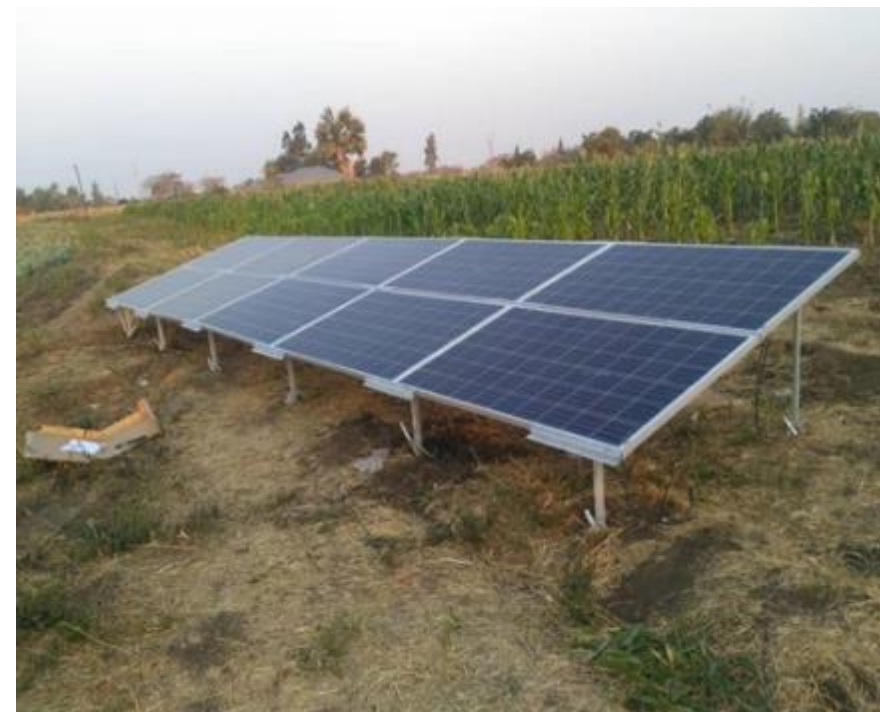
Picture of Solar Water Pump Irrigation
