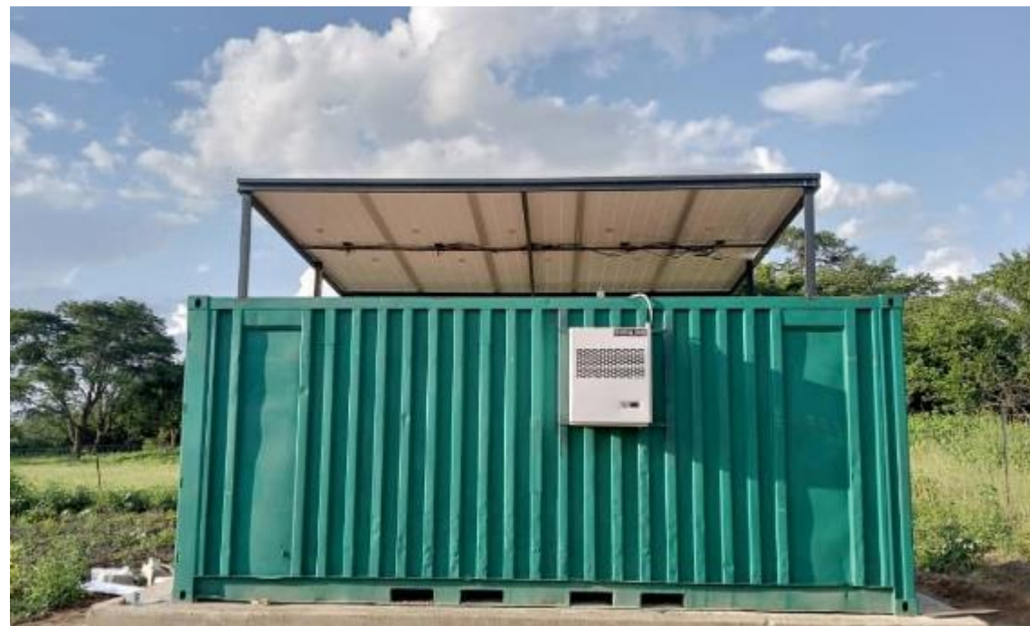
Solar Cold-Room in Nangoma - Mumbwa
