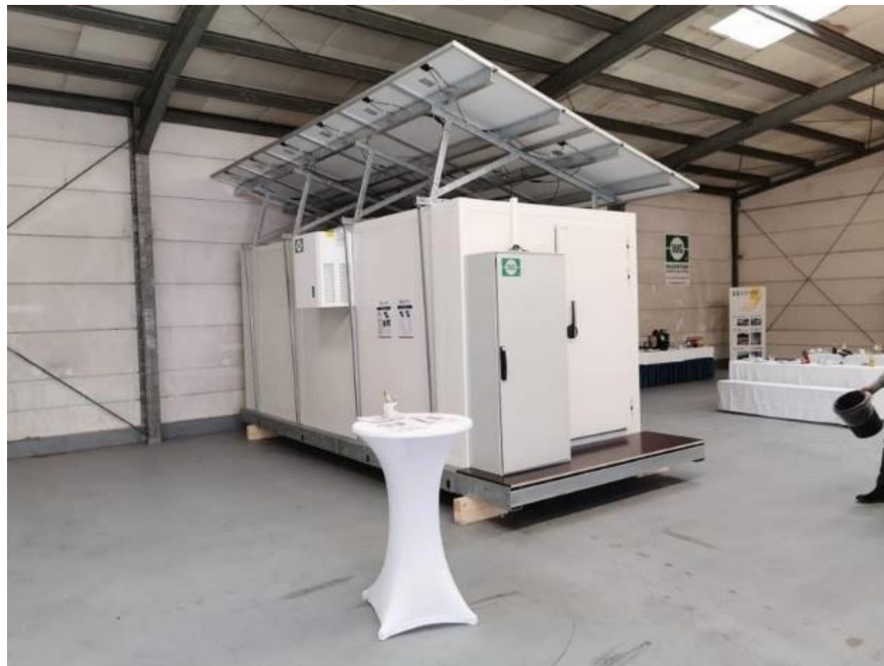
Picture of a Solar Cold-Room within a building
