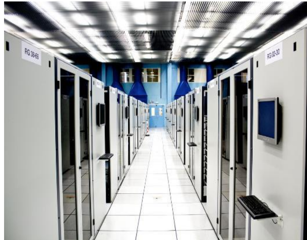
Picture of Data Center IT Cooling Solution
