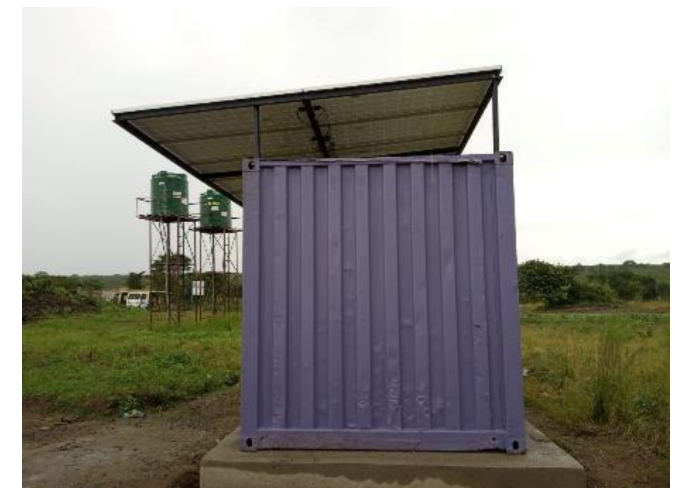
Solar Cold-Room at St Paul's - Kabwe
